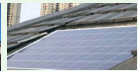
Standard solar PV panel (polycrystalline silicon)
